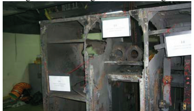
Damaged breaker arrangement at a switchgear
