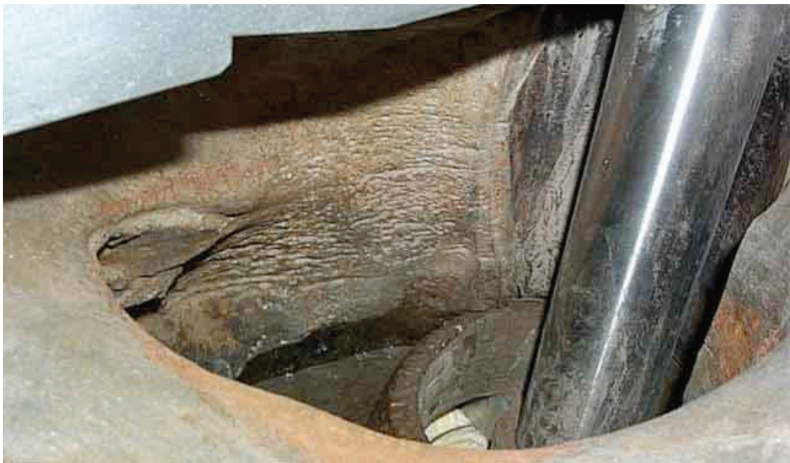
The large hole in the reactor vessel head around the vessel head nozzle.
