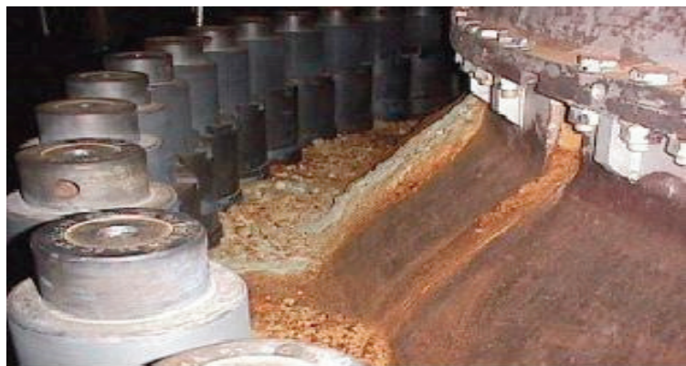
Rust-laced boric acid "river" flowing through inspection ports on the reactor head and down onto the reactor flange during the refueling outage in 2000.
